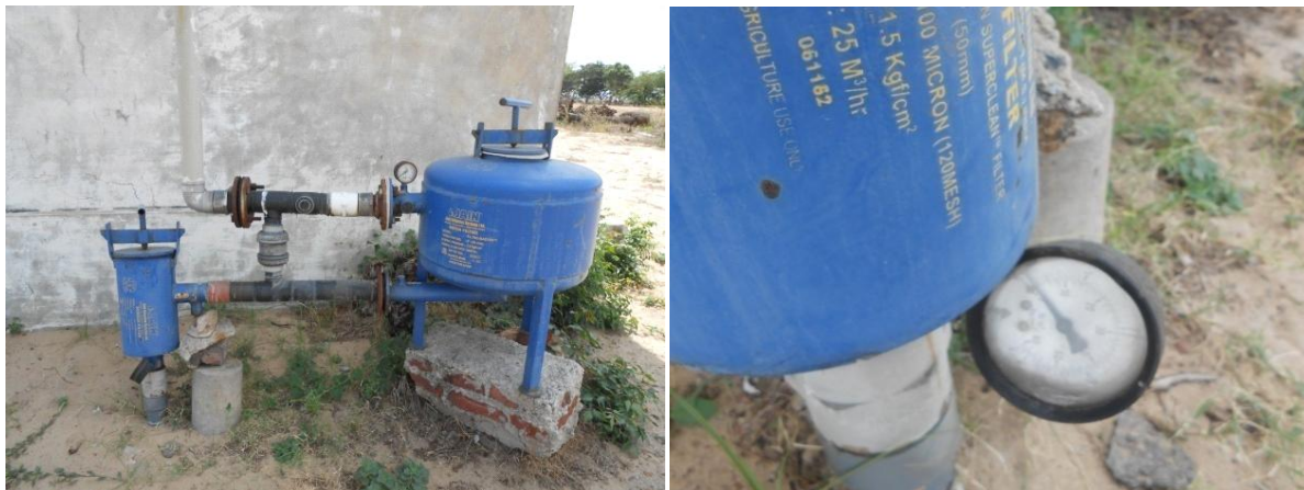
Plate 1. Water distribution system with sand filter, screen filter and other accessories
